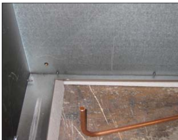
Gas supply pipe under bottom of gas control box.
